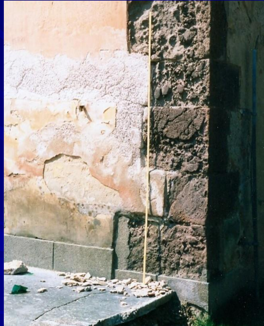
Patterns of efflorescence both on rocks and on mortar
