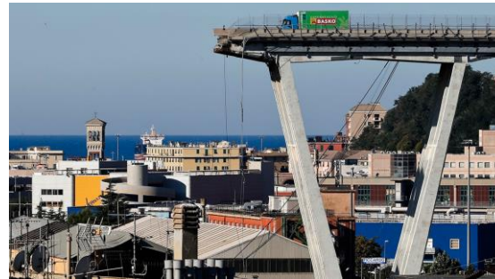
Ponte Morandi in Italy
